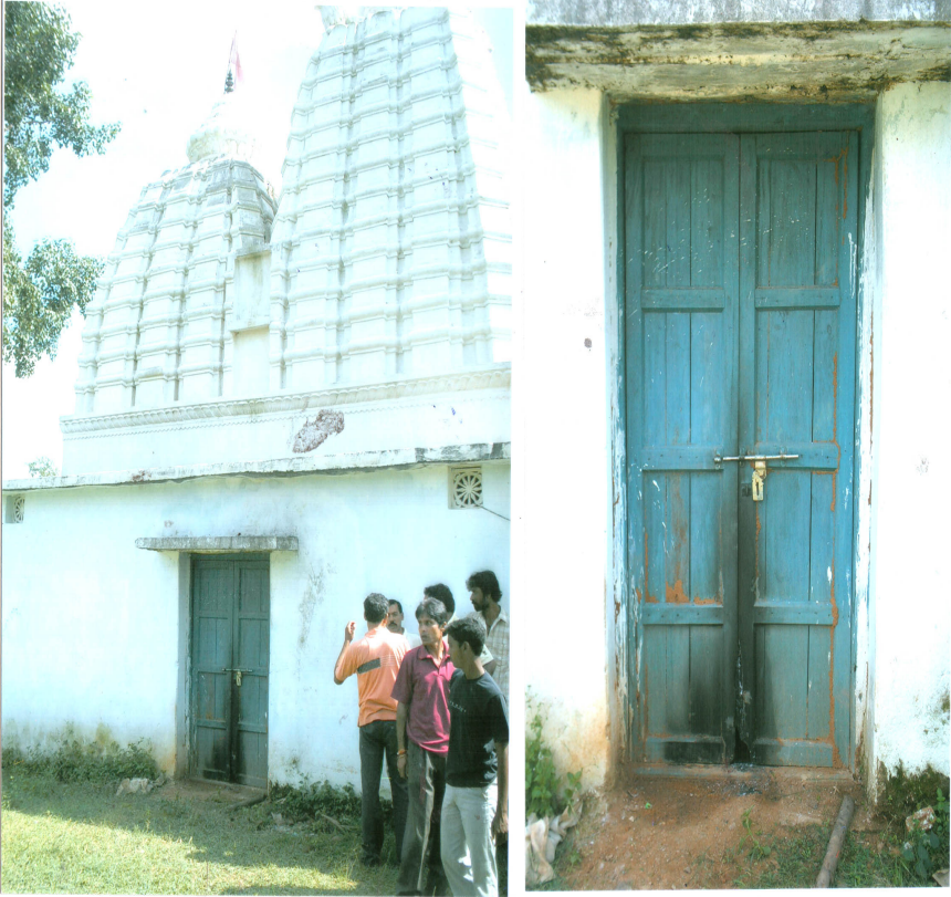
Hindu Temple Door Charred by Fire
